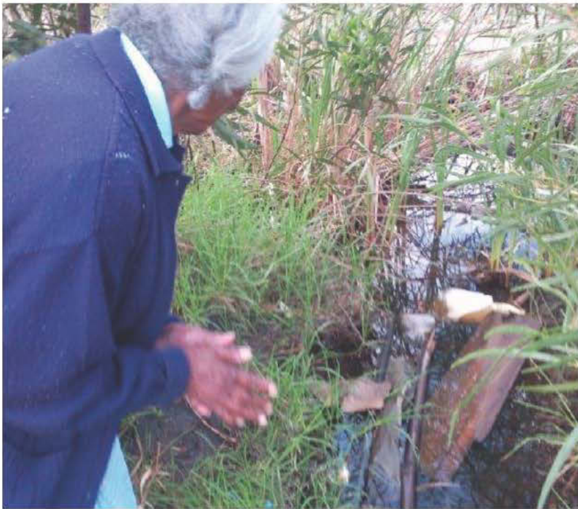
SFP client Mrs Klaasen shows LHR staff members the faulty water connection near her home
